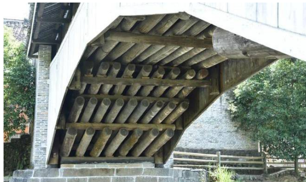
Fig. 1. Stacked Wooden Arch Beam Structure of Puji Bridge in Pingtan Township, Hunan.
